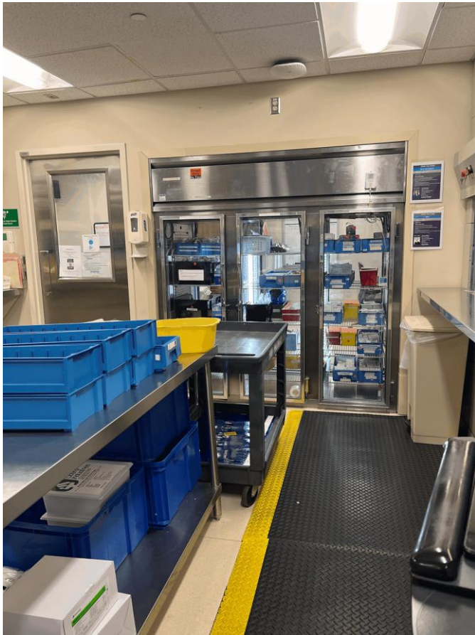
Outside the Ante room where some supplies are located and refrigerated med
